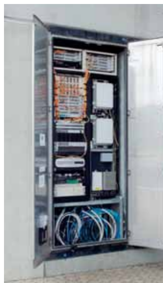
Equipment rack serving one of the speaker zones
