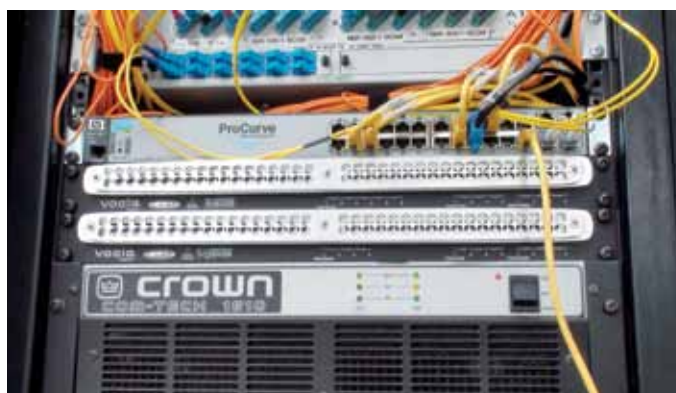
VI-6 and VO-4 units in situ
